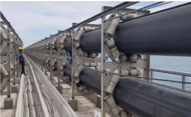
PIPE CONVEYORS, EACH OF ABOUT 9.5 KM LONG, TO TRANSPORT UNLOADED CARGO DISCHARGED BY BERTH CONVEYORS TO SHORE
